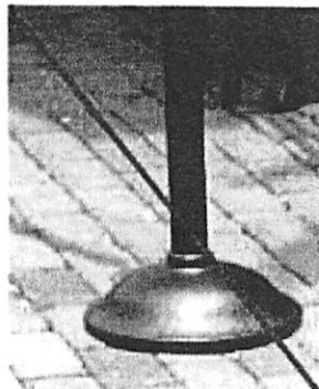
FIGURE 5 Domed stanchion bases are not permitted
